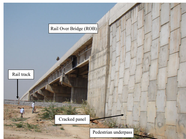
Fig. 1 Misalignment of the reinforced earth wall close to the rail over bridge
